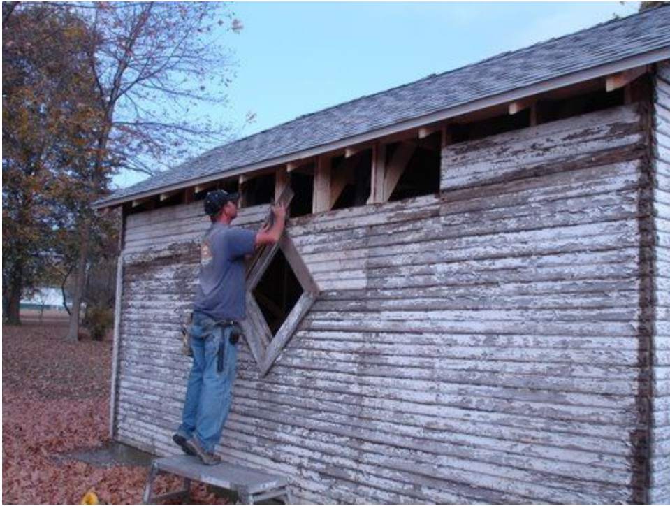
Repairing the south side of the garage. Rotten siding had to be replaced.
